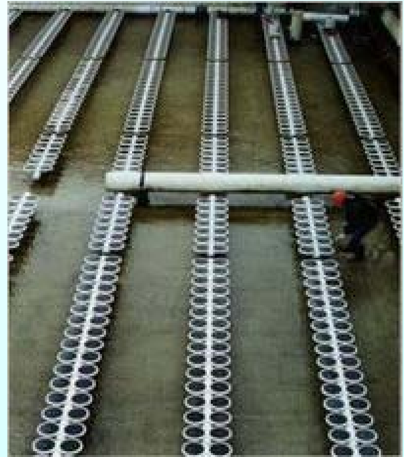
Fine bubble membrane diffusers in an aeration tank
